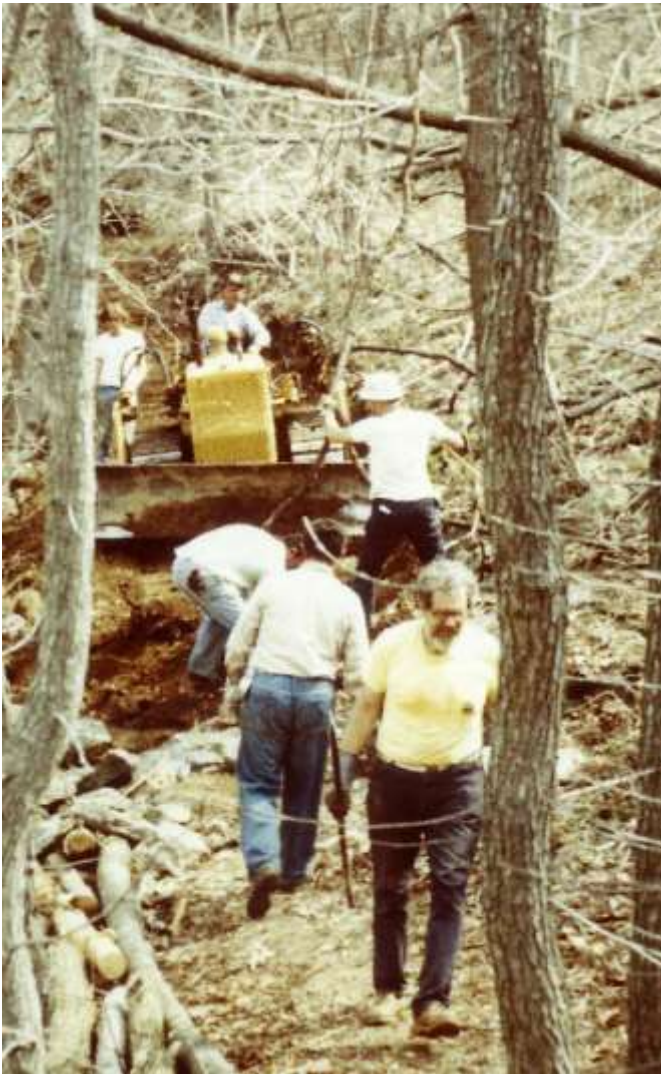
Winter 1979 - Harold Crate and others create part of the access road to the cabin site - someone brought their bulldozer
