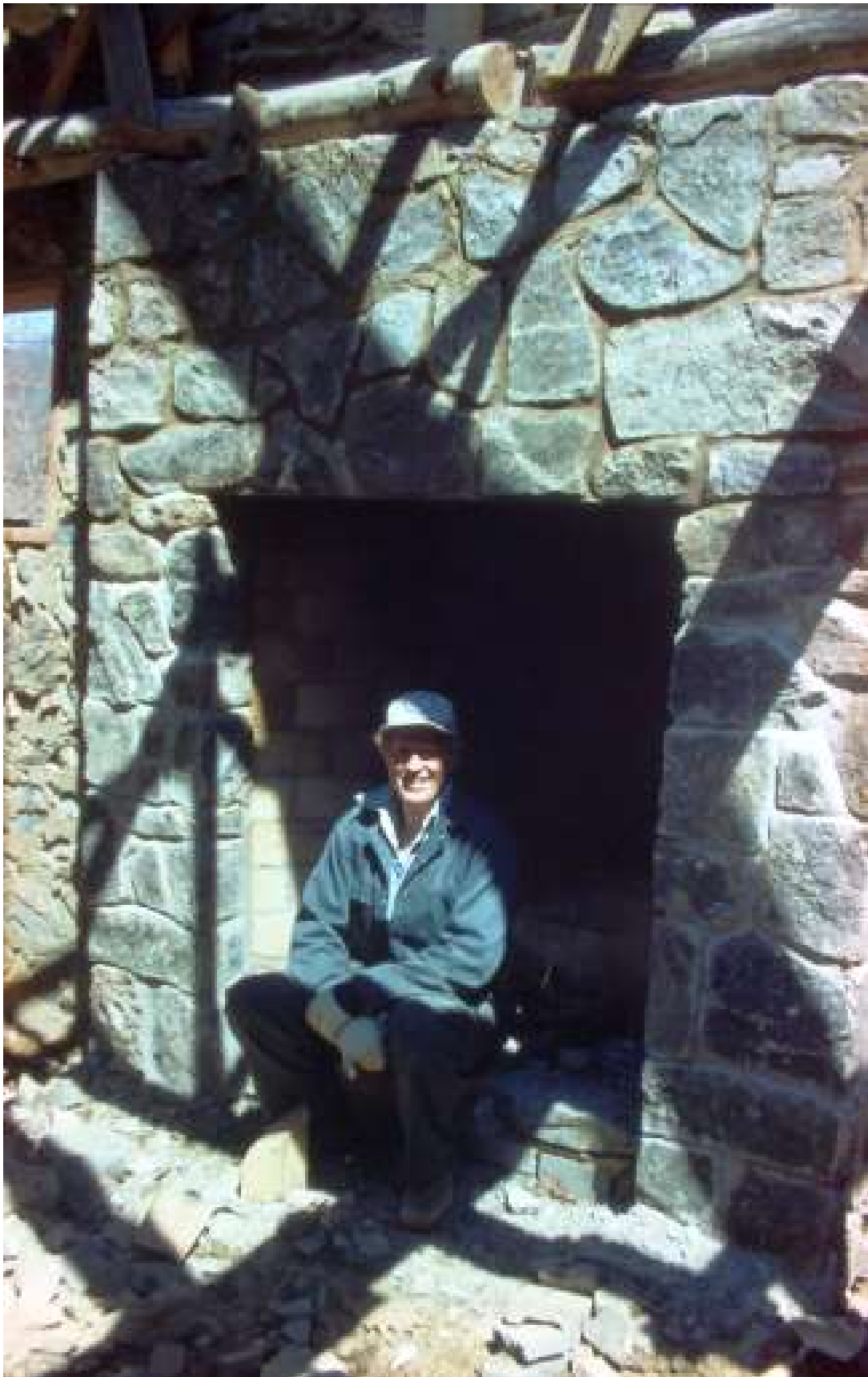
April 1982 - Otey Shelton supervised the laying of stones - He did the work on the fireplace himself
