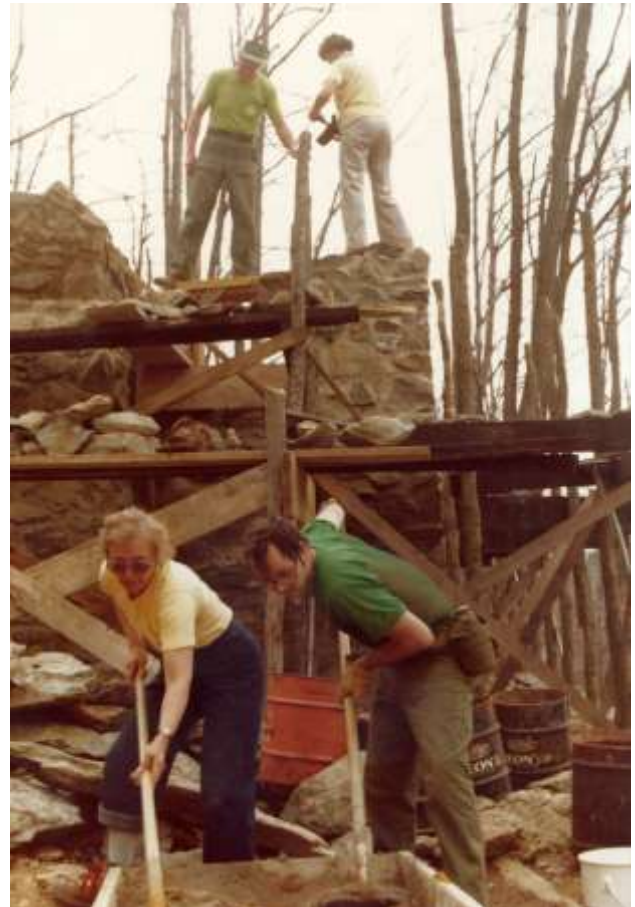
April 1981 - Otey and Margaret stand atop wall while Lee Hulten and Ken King mix mortar below
