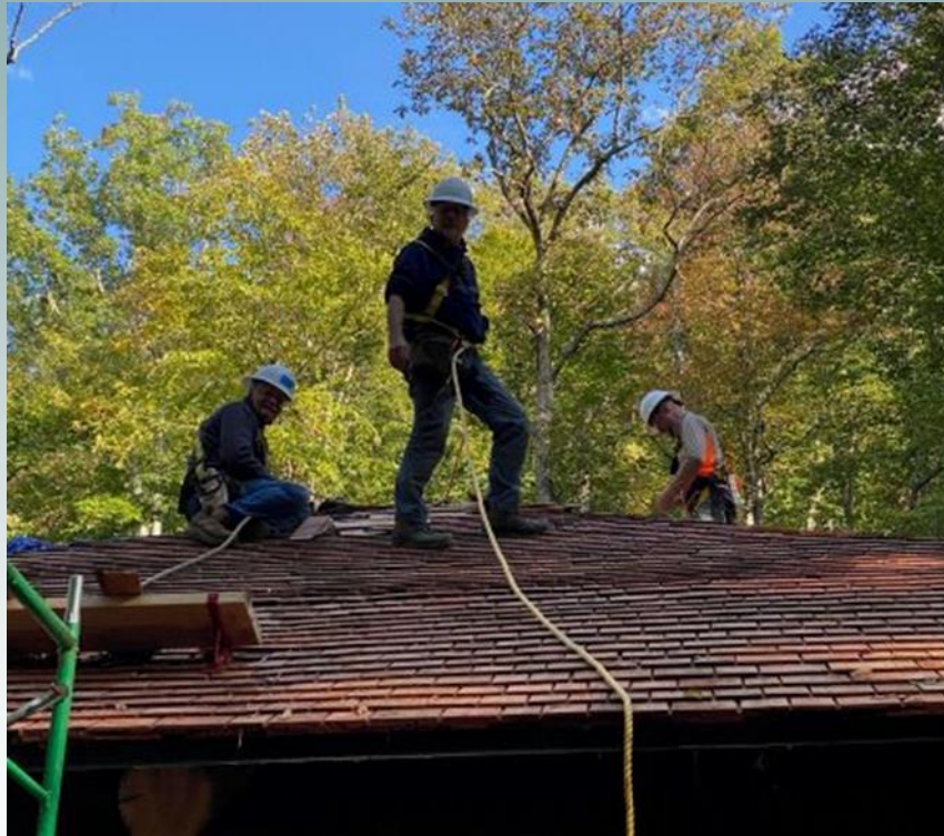
Pete in the center standing on the roof (early October session). The team finished the east and southeast side of the roof, ripping out shingles and purlins on the southwest side.
