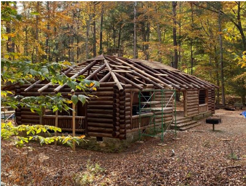
Rotten shingles and purlins had been removed (early November session). This is the north facing side of the pavilion.
