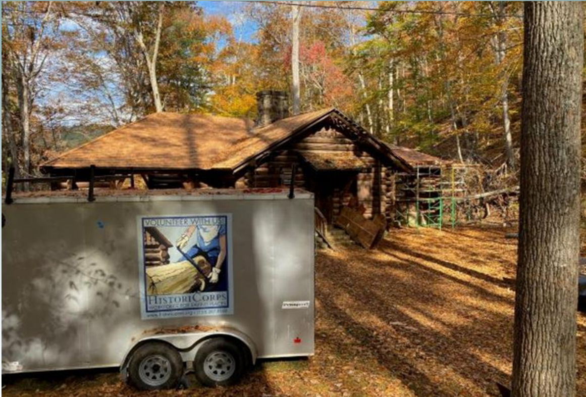
Tool trailer and view of the back of the pavilion. The southeast side (left) has a kitchen inside the pavilion. The southwest side (right) shows scaffolding and is where a lot of the rotten purlins and the rotten main rafter was found.
