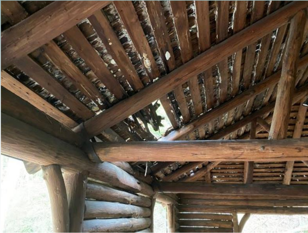
North side of the roof as it appeared when Pete first showed up. Fungus was growing on the bottom of the purlins and shingles (see white spots) where all the water was leaking through.
